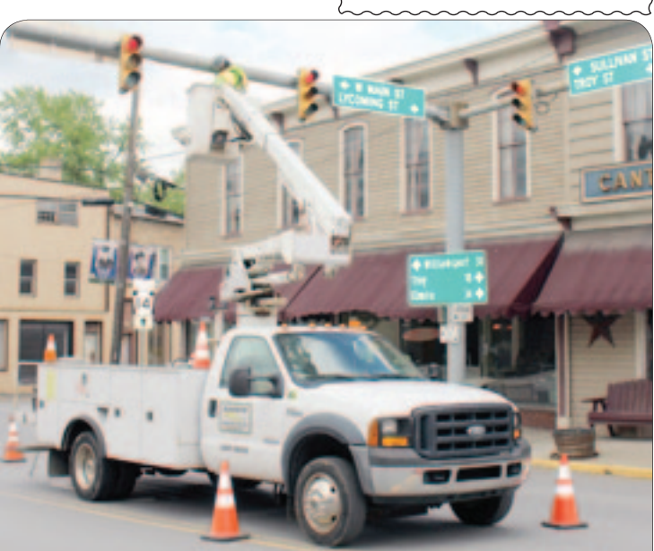
Canton was awarded an ARLE grant to be used to re-do the traffic lights, parking areas, stop bars, etc. at Canton's Main Square. The work has been underway for a couple of weeks.
