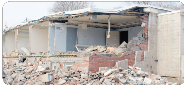
If you drive past what used to be the Troy Hospital, you will see that it is currently being demolished to make room for the new Dollar General.
